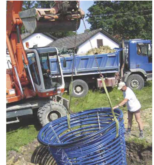
Geothermiekorb; Quelle Rhein Ruhr Collin AG
